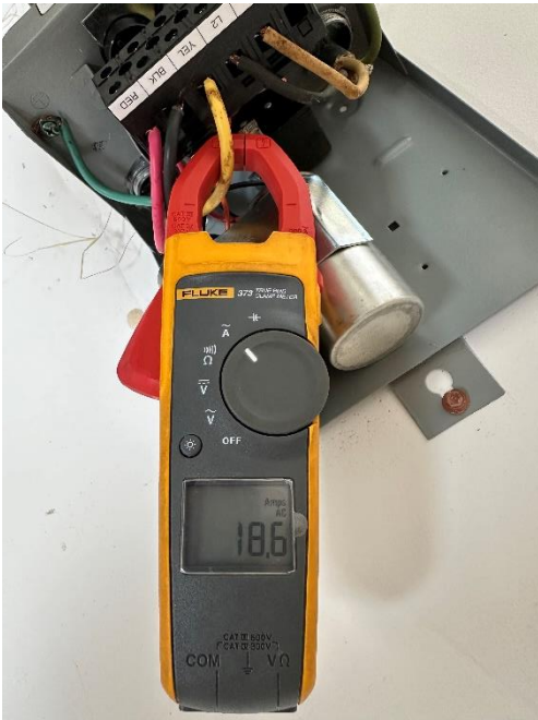
Running amperage of well pump
