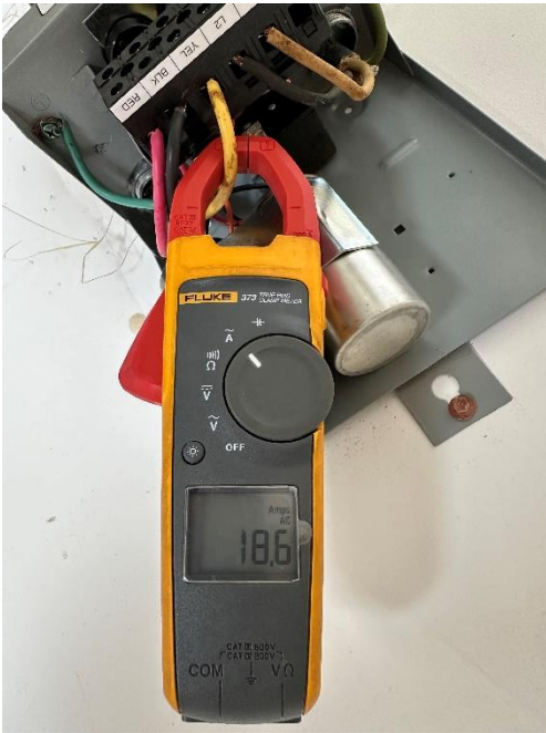
Running amperage of well pump
