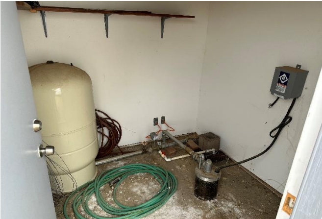
Well head Pressure tank and Control box
