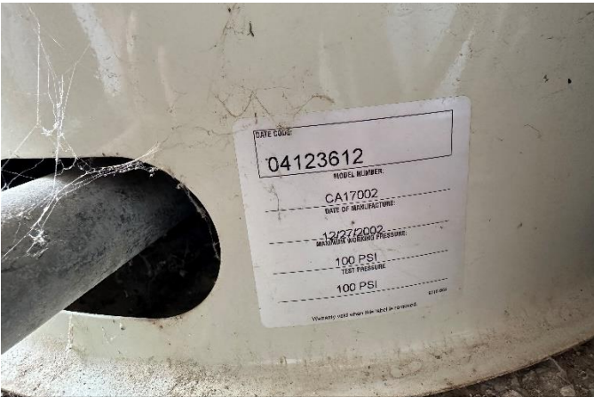
Pressure tank date code sticker
